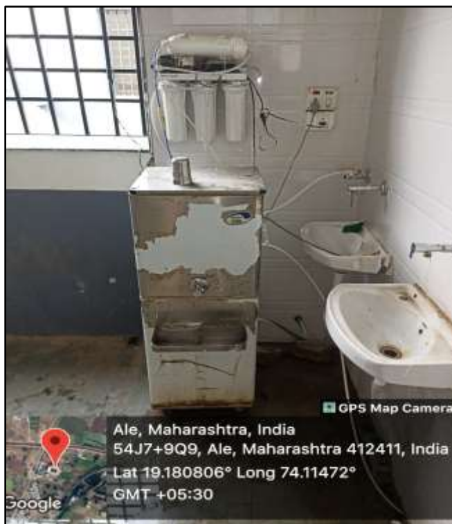
Drinking Water Facility in Campus
